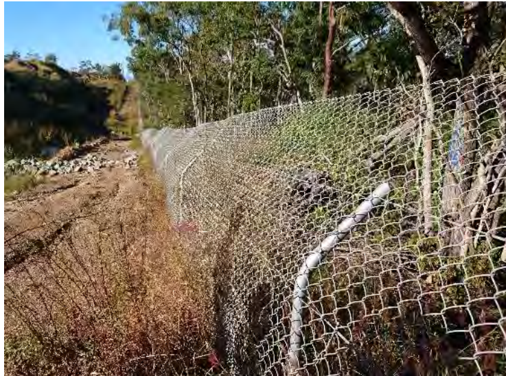
Figure 6. Koala barrier fencing erected in association with the upgraded Eton Range upgrade of the Peak Downs Highway.
