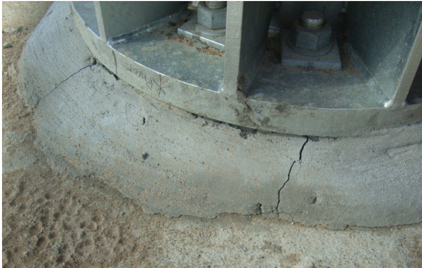
Figure 1 – Reflective cracking indicates the mortar is not sound
