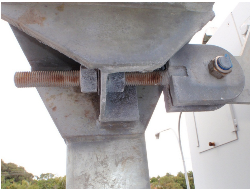
Figure 26 – View of the poorly fabricated clevis bracket
