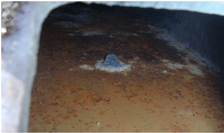
Figure 40 – View of the lack of zinc coating on the inside of the top member
