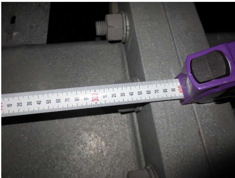
Figure 23 – View of the distance available from the first vertical member to the splice joint
