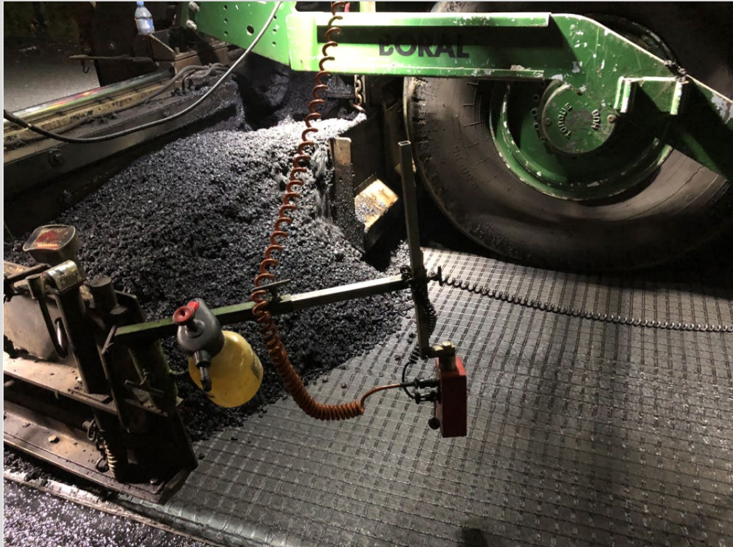
Figure 9.7.1 – Example of asphalt being paved on asphalt geosynthetic with no bow-waves, wrinkles or folds
