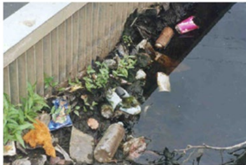
Figure 3.5.7(c) – Trash rack and pollutants
