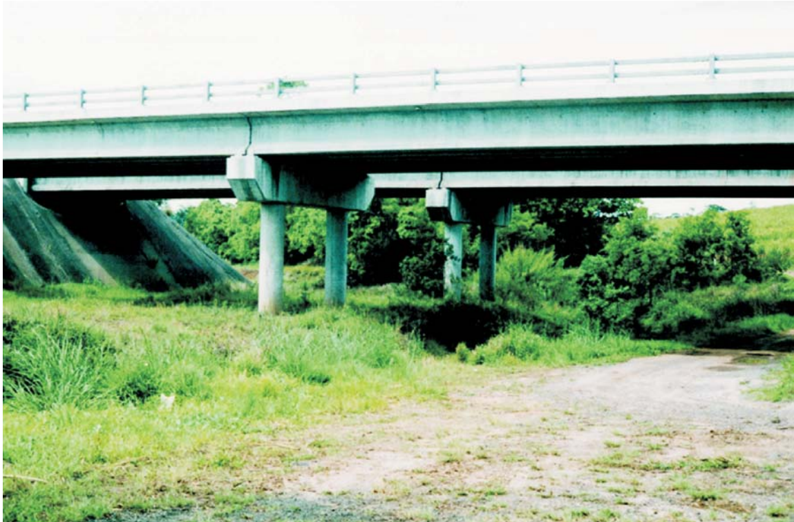
Figure 6.3 Ideal opportunity to provide native plantings under a bridge that has dry fauna passage (Nambour Bypass, south-east Queensland)
