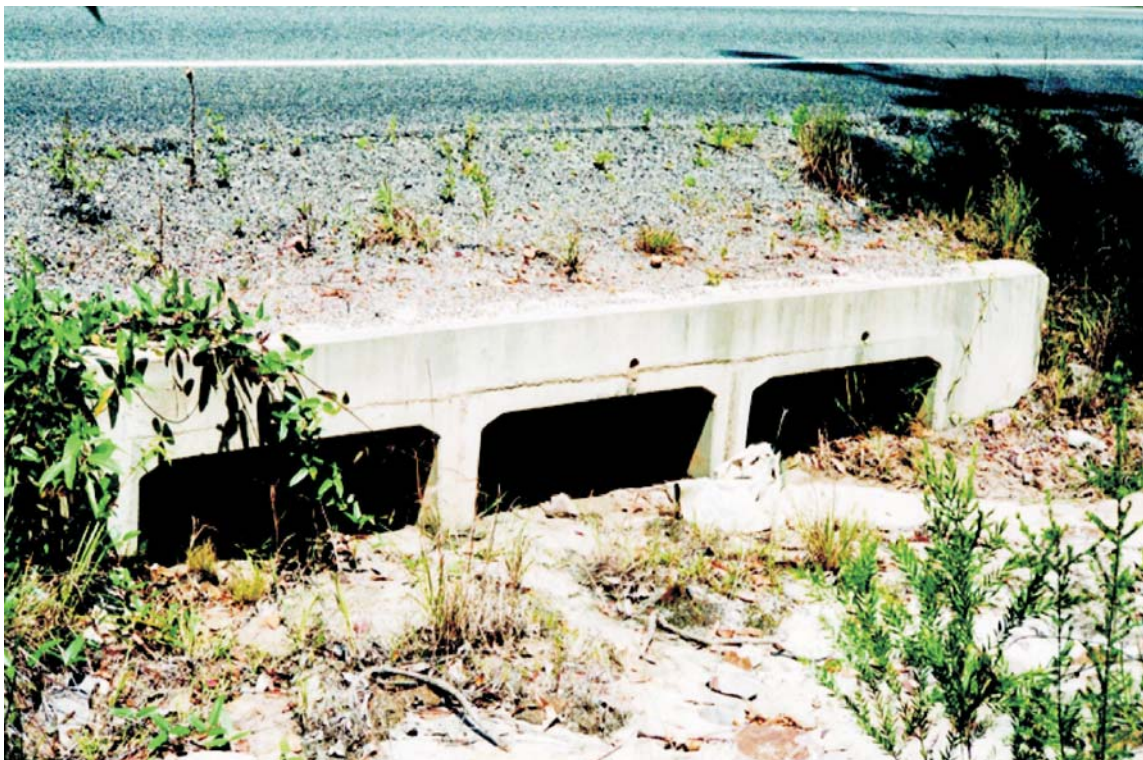
Figure 6.6 A small three cell box culvert partially obstructed with sediment and with little revegetation of entrance (Sunshine Coast Motorway, south-east Queensland)
