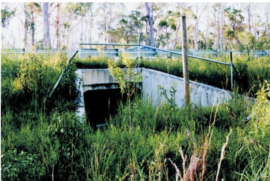
Figure 6.10 A Koala refuge pole located outside a well revegetated culvert entrance (Brunswick Heads Bypass, northern NSW)
