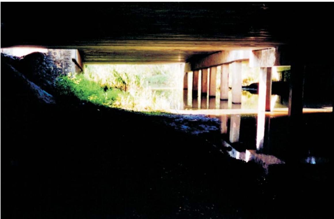
Figure 6.4 Bridges which are dark and have limited dry passage for fauna, consequently providing inadequate cover for native fauna species (Bruce Highway, south-east Queensland)
