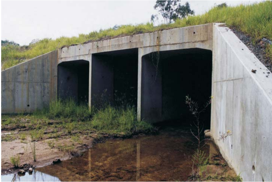
Figure 6.9 A culvert in which accumulated silt provides a substrate for revegetation but exotic species dominate (Burnett Highway, south-east Queensland)
