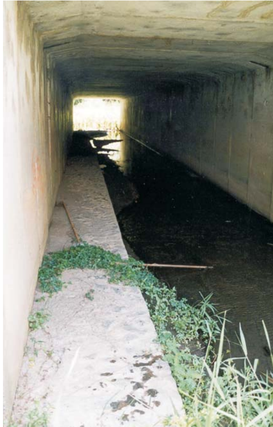
Figure 6.5 Raised ledges within a culvert (Old Northern Road, south-east Queensland)
