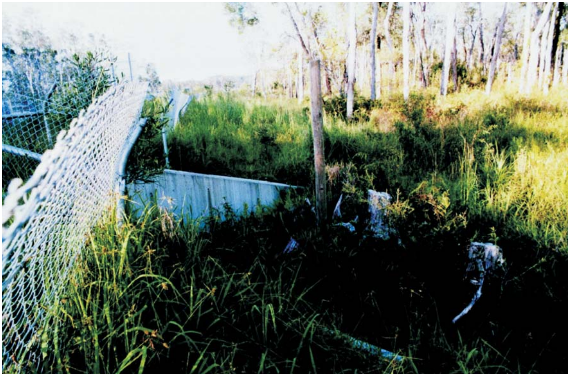
Figure 6.8 A culvert entrance where revegetation of native species is well advanced, providing good cover for fauna (Brunswick Heads Bypass, northern NSW)
