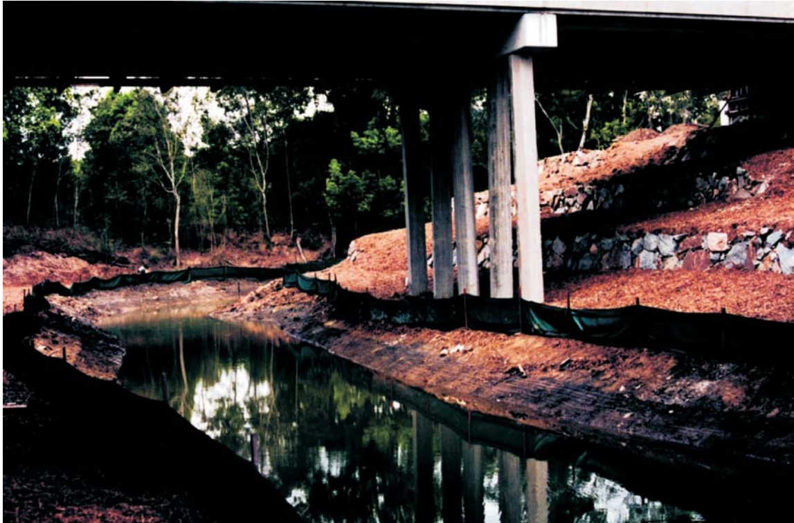
Figure 6.1 Steggalls Creek bridge on the Yandina Bypass, south-east Queensland, shortly after construction (1997)
