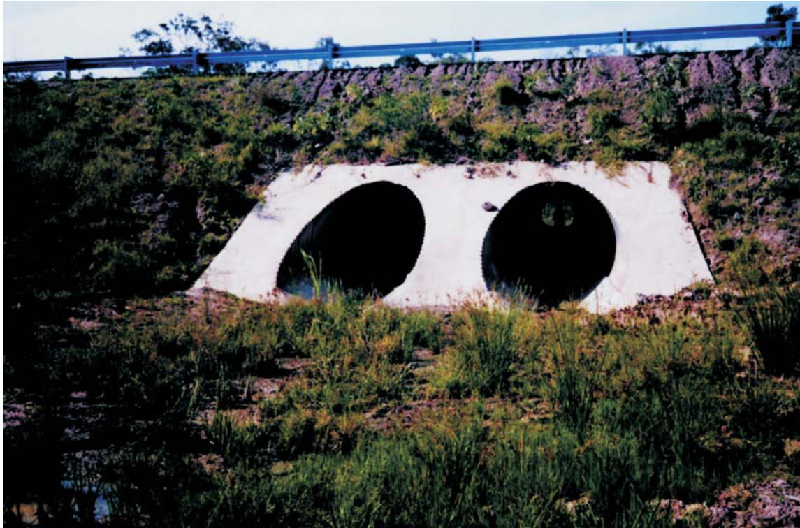
Figure 6.7 Pipe culverts where limited revegetation provides little cover for fauna (south-east Queensland)
