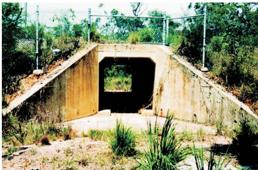
Figure 6.13 A culvert with wildlife guide fencing and raised ledges (Sunshine Coast Motorway, south-east Queensland)
