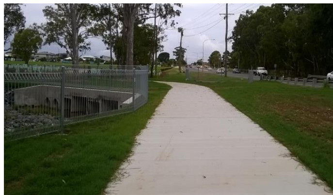
Figure 4.2(B) – Example of good fence placement where the fence borders the hazard and is set back from the path
