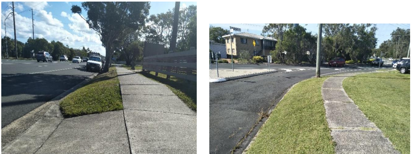
Figure A5 – Batter slopes adjacent to paths may propel users towards hazards
