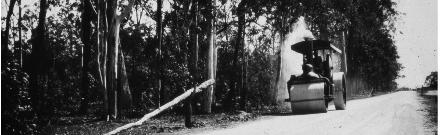
Section under construction steam roller operating on dirt section of Redcliffe Road.
